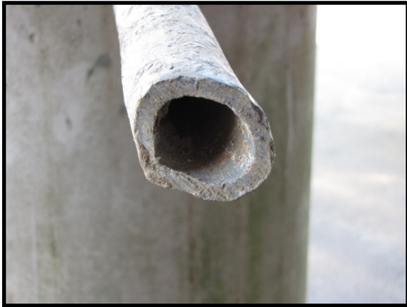
Lead Service Lines (Stopped use in 1950's)
